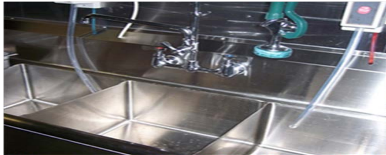
Figure 21. Three (3) Compartment Sink with Backsplash
